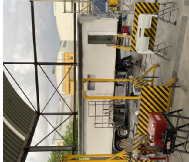
NINOX production floor with the semitrailer under equipment installation. In the foreground, the electrical generation system and NINOX precision welding equipment.
